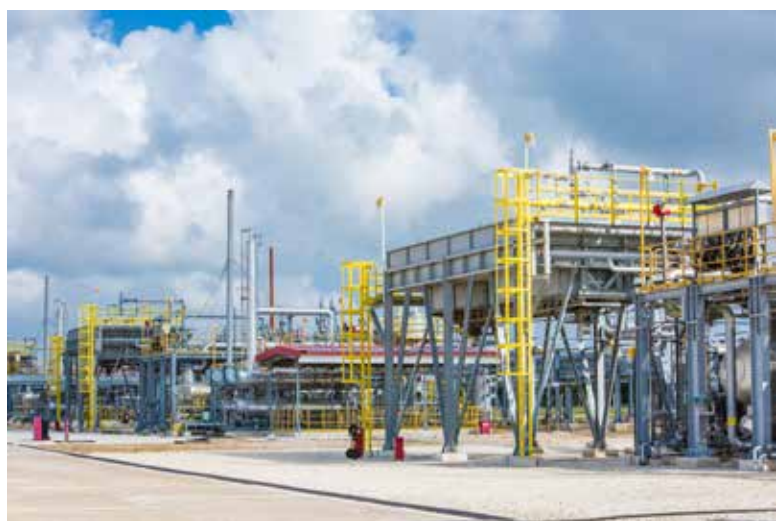
Gas Processing Plant, Madimba Mtwara
